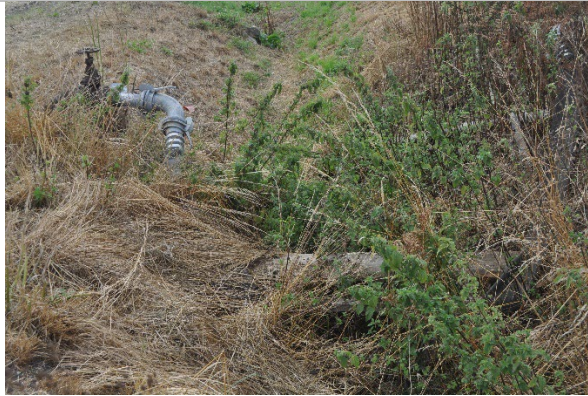
Plate 33 Permanent pipework on the channel bank
